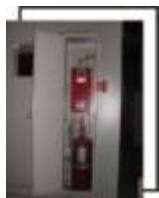
Fire Suppression System
